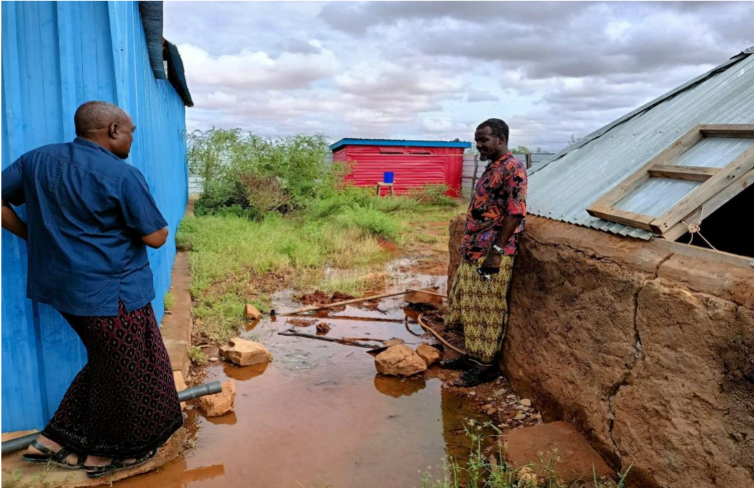
Figure 3-10: Underground water tank with Pit latrine ( in red corrugated iron sheets) at the far end. entrance in the background
